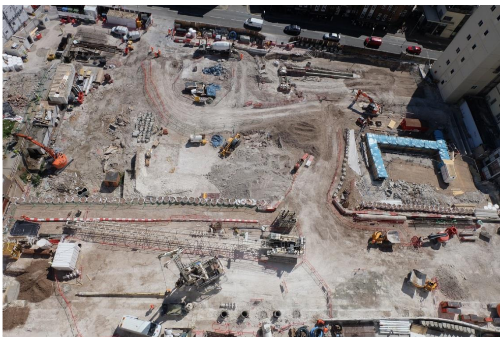
An aerial view of the Stage 1 site with the piling rig working at the bottom (north side) of the picture.
